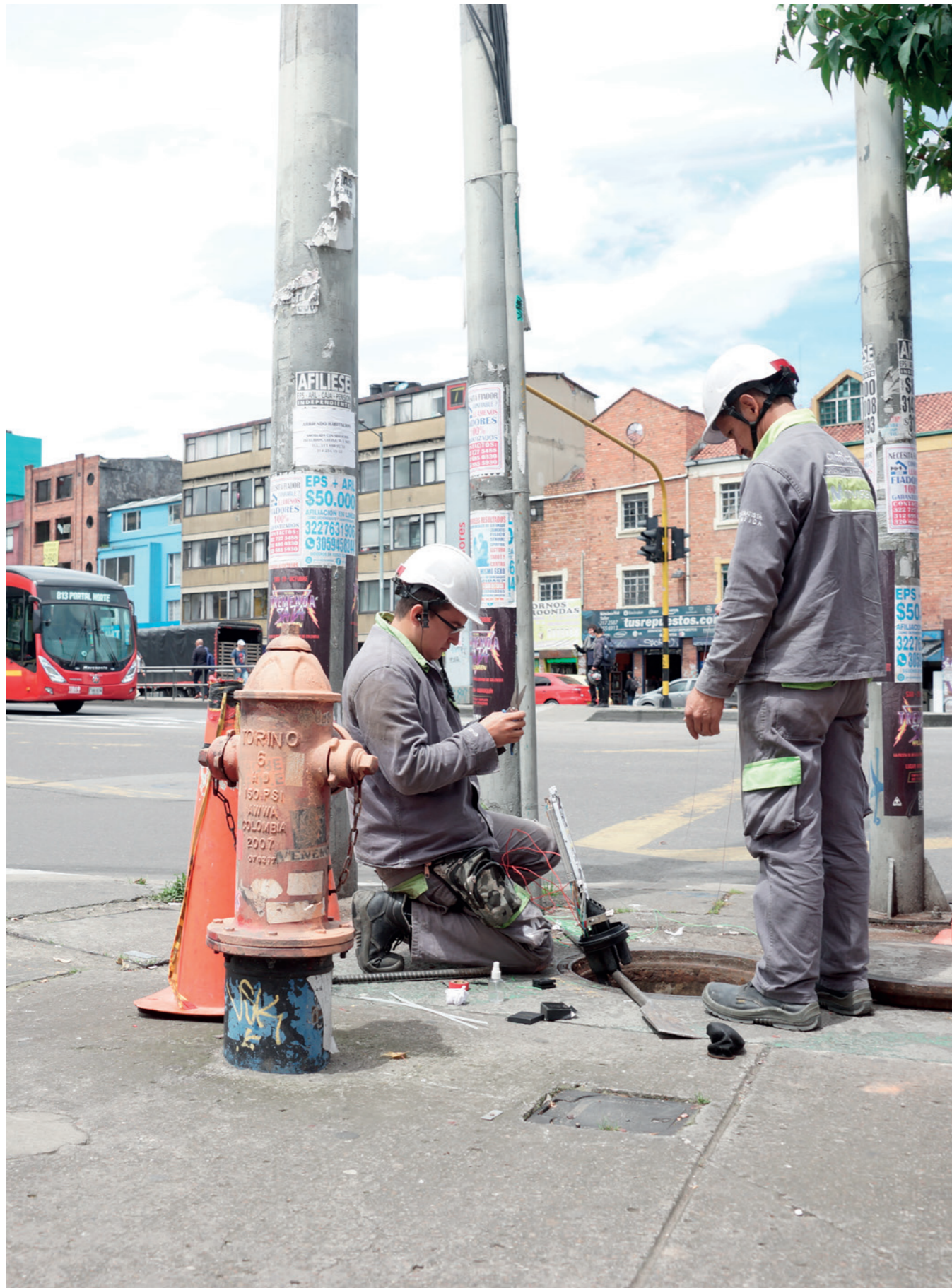
Street repairs in Bogotá, Colombia. We currently work with seven Swedish companies and their supply chains in Colombia. The workplace committees we work with cover topics such as diversity and inclusion, women empowerment and human rights, which contributes to improving employer-employee relationships in Colombia.
